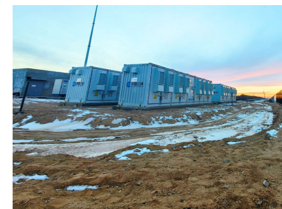
Mazongshan 50MW PV storage project
